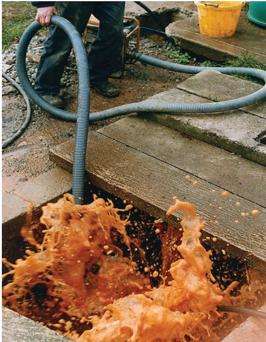
Airlift surging and pumping to clean iron oxide and ferrophyllic biofilms clogging a Local Authority water supply borehole lined with slotted mild steel casing. The slimy biofilms had clogged the slots in the steel and the small water bearing fractures in the rock. The borehole was pumped until clean and the sustainable pumping rate had increased from 36 to 340 cubic metres per day
