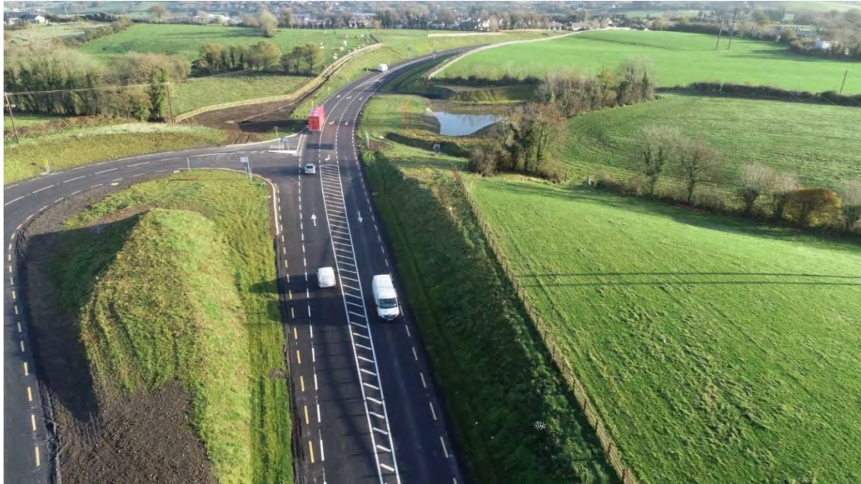
Above: An aerial view of the realigned N55 at Garrymore, and the new junction with the L-6552, complete with dedicated right turning lane.
