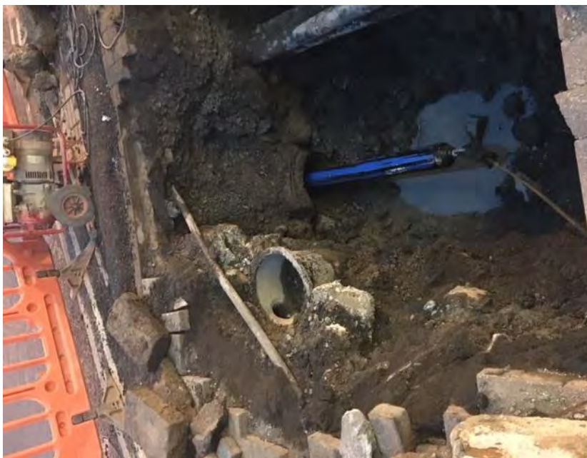
Slip Lining 125mm pipe through 200mm Asbestos pipe on footpath near to post office footpath.
