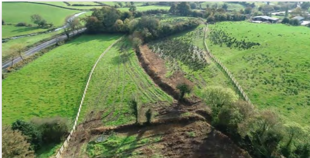
Above: Aerial views of the boundary fencing works on the N55 Corduff to South of Killydoon Realignment, Section B at Ballytrust
