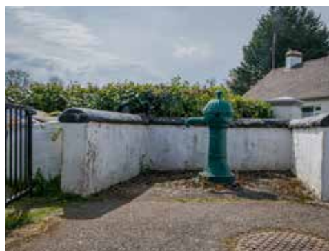
Fig. 19: Cast-iron water hydrant detached house located in Butlersbridge.
