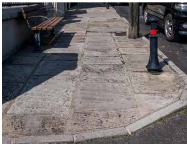
Fig. 16: Paving slabs outside the courthouse.
