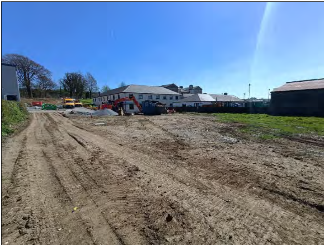
Figure 14. Overview of disturbed bare ground in north area of site near school
