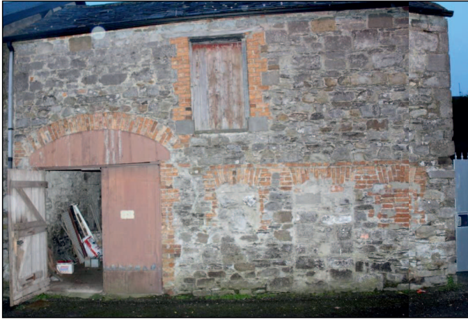
Plate 6: Two storey stone structure at rear of PDA facing on to Patrick Street
