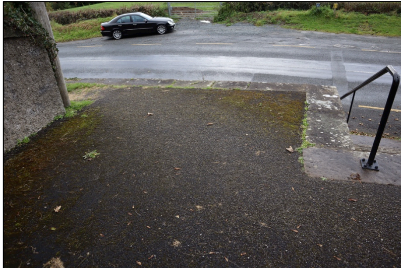
Figure 10: Tarmacadam surface at steps and leading to entrance gates
