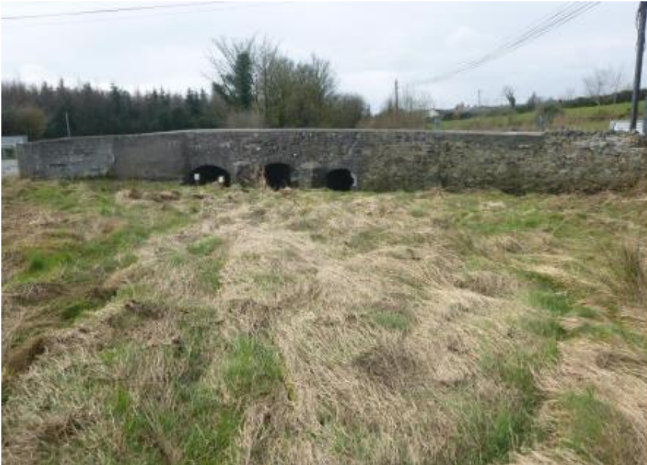
Photo 3 – area upstream of Assan Bridge where new bridge will be constructed. The course of the river will be altered so that it approaches the bridge directly as opposed to the current situation where it approaches the bridge from the north-west and flows along the bridge wall before turning south under the bridge.
