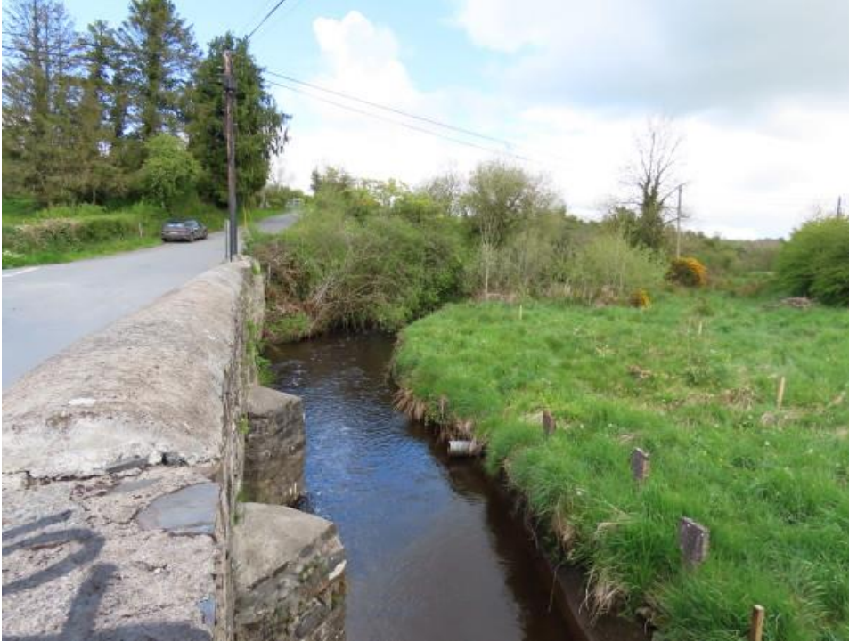
Photo 2 - view of watercourse upstream from bridge showing current course of river. The course of the river upstream of the bridge will be altered so that it flows directly under the bridge
