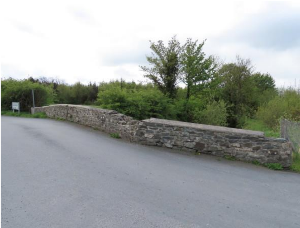
Photo 7 – Downstream parapet wall with damaged section
