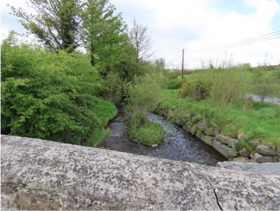
Photo 8 – view downstream from existing bridge showing rock armour on western river bank
