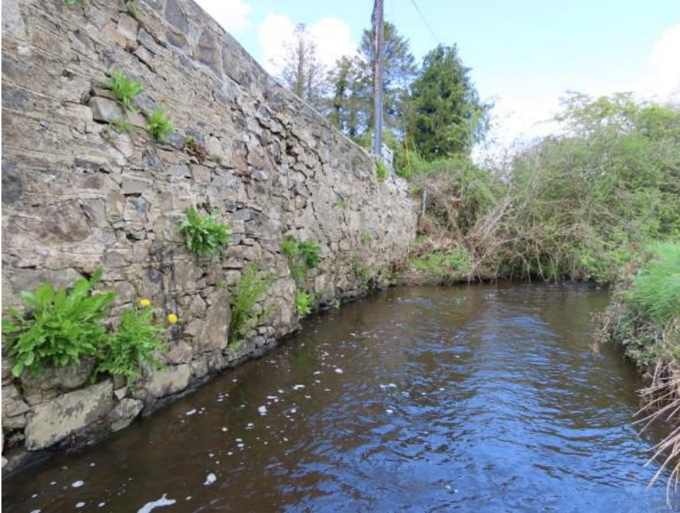
Photo 4 - cracked masonry wall upstream of bridge. Watercourse flows along this wall before turning south under the bridge.
