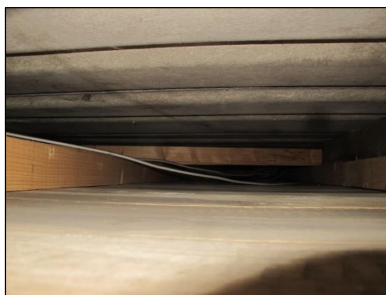
Plate 4. Space between sheet metal roof (above) and cladding (below) is not insulated
