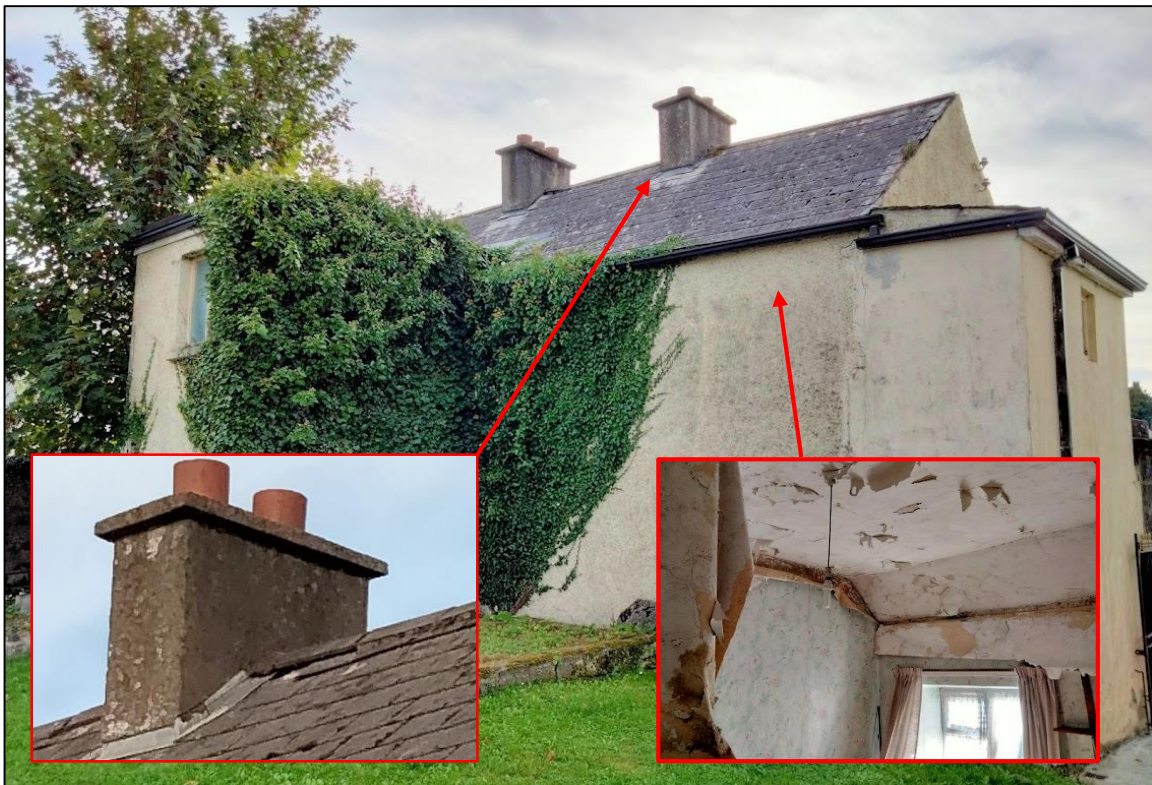
Plate 7. Rear of 16 Abbey Street. Roof has potential bat roost features around chimney flashing and ridge (inset photo). Building suffers from damp with apparent water ingress of rain through roof with ceiling plaster deteriorating. Ceiling has no attic hatch and roof space could not be surveyed. Water storage tank is located on flat roof at rear of house. Photo facing south-west
