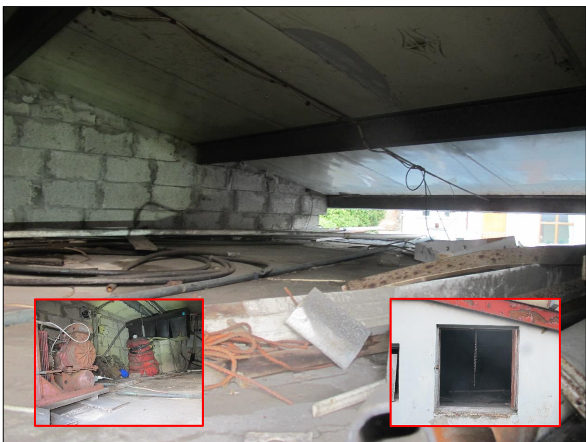
Plate 11. Donohoe's Foodfare machinery housing. Inset photos of machinery and services (left) and west facing hatch (right) where two bat droppings were noted.
