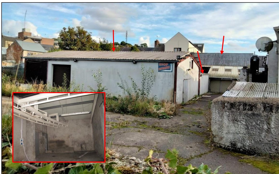
Plate 9. Rear of Donohoe's Foodfare buildings, marked with red arrows. Inset photo of meat processing room. Photo facing south
