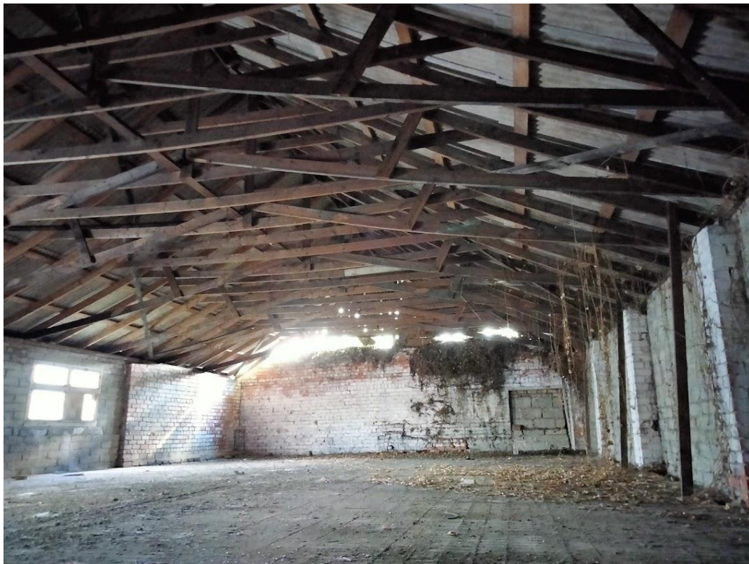
Plate 16. First floor of Back Building. Survey of this space was not possible due to floor in dangerous condition with wall plate supporting the floor coming away from wall bulging outwards (on right/back wall). While no bat roost features were discerned from a vantage point in the north-west corner (as per photo) the building is open at the southern end and there is potential for night roosting/perching in the roof timbers. Bats were not observed emerging from the Back Building during surveys.
