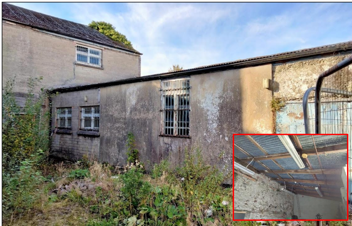
Plate 17. Right Annex off Back Building. A dead startling was noted in this section which connects with the Back Building. No likely access points for bats were noted. Inset photo of internal roof space
