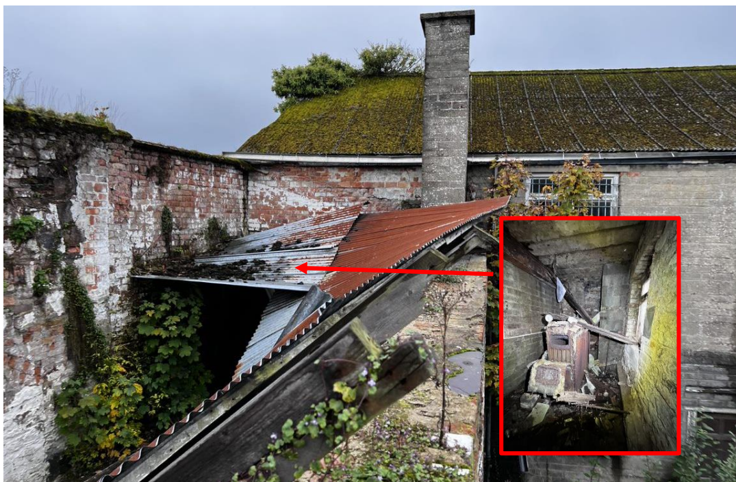
Plate 19. Left Annex, roof facing onto the front (north) has collapsed, rooms below are exposed and damp. Photo by Liam O'Reilly, Architect (Cavan Co. Council)
