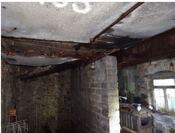
Old Boiler, First Floor Over, C
