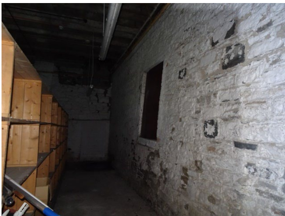
Ground Floor Western Wall Building A Out of Plumb
