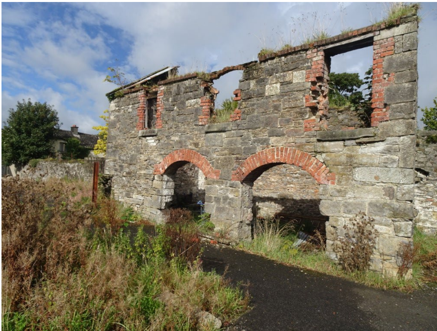
Southern Elevation with Brick Arches Flimsy First Floor Window Lintols
