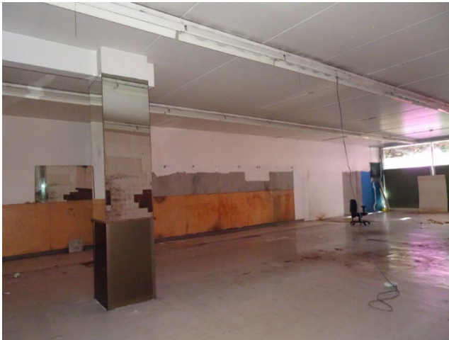
Single Storey Area with Wide Span Precast Concrete Roof, Central Column Supports Transfer Structure Over
