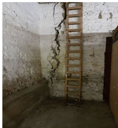
Crack in Northern Wall 2019 A
