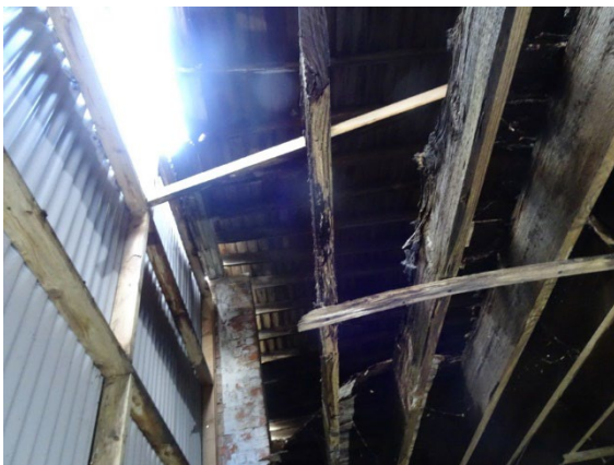
Flat Roof Section Roof Failure, South wall Metal cladding, and First Floor Joists Decayed B
