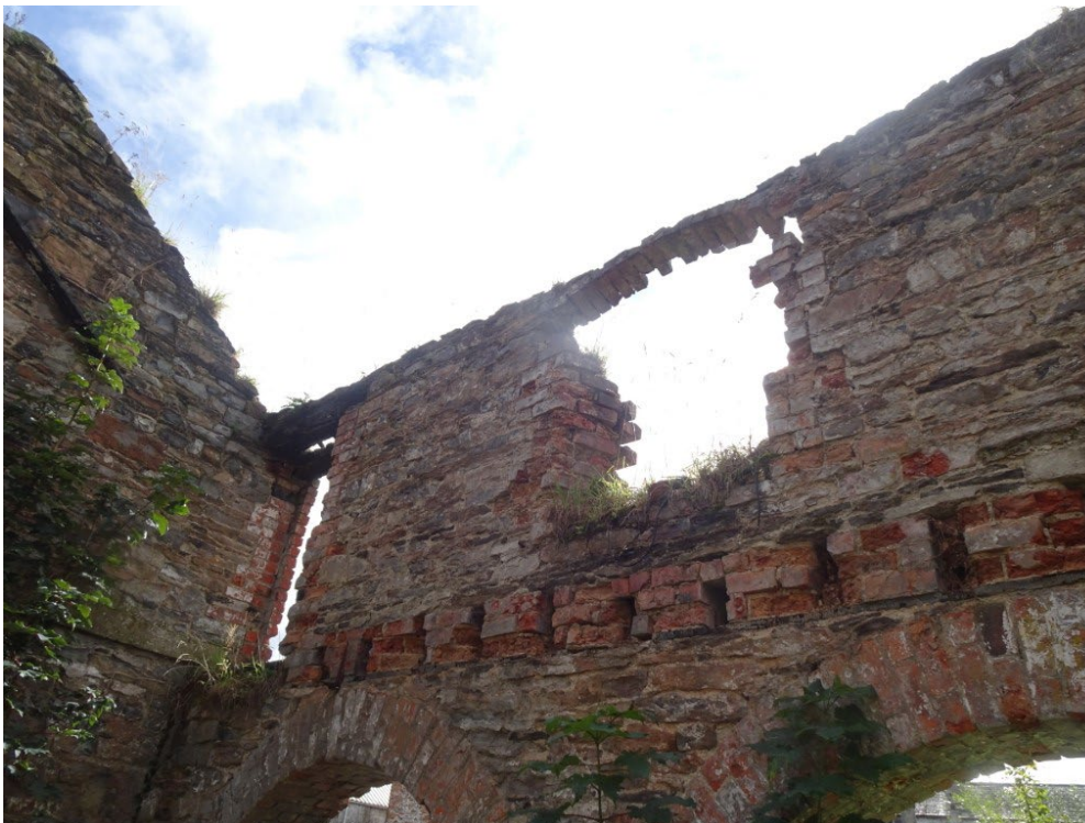
Internal View of Southern Wall With Brick Courses at First Floor Joist Level, Precarious Brick Arch Over First Floor Window
