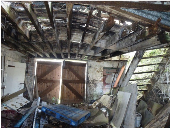
Area Inside Double Door, Roof Collapsed, Floor Joists Partially collapsed, Floor Debris, C
