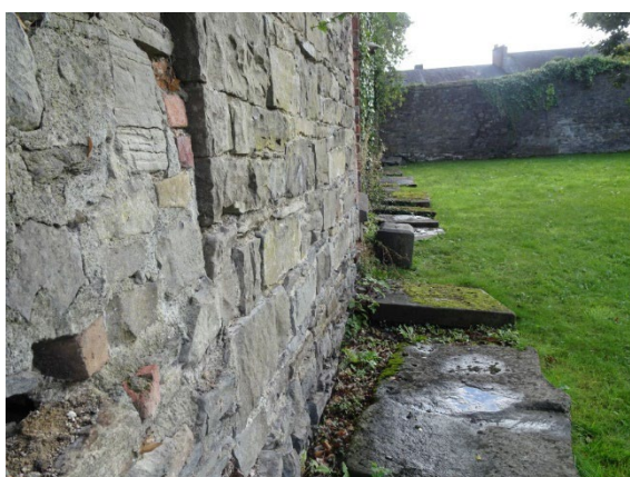
Western Wall Misaligned and Out of Plumb A
