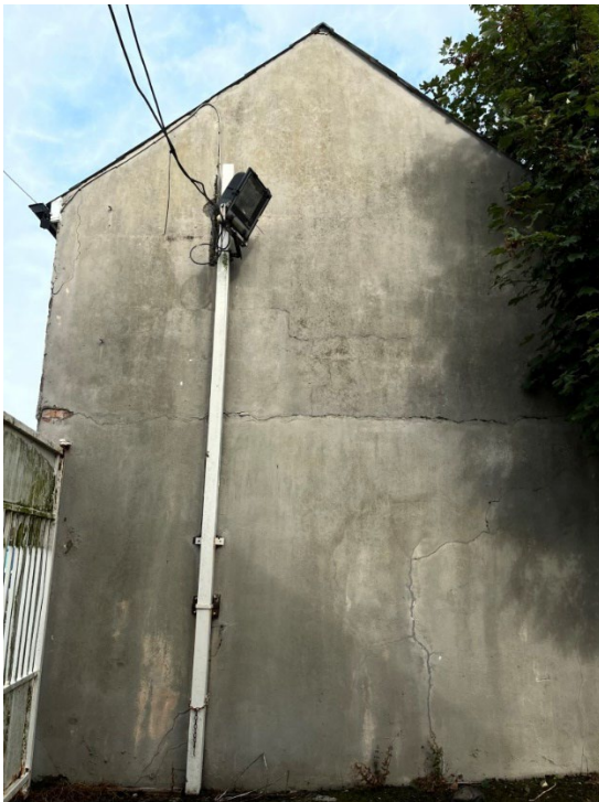
Southern Elevation with some Plaster Cracking but is in quite good condition
