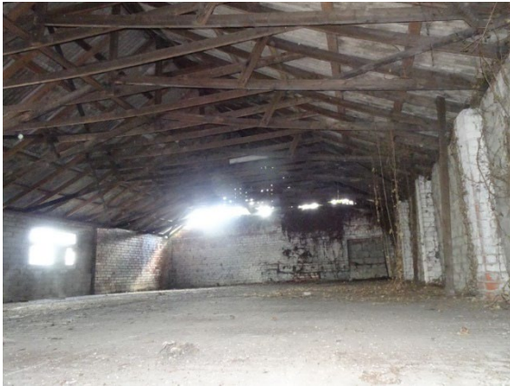
First Floor showing Timber roof Trusses, Holes in the Roof and Piers on the Western Wall, A
