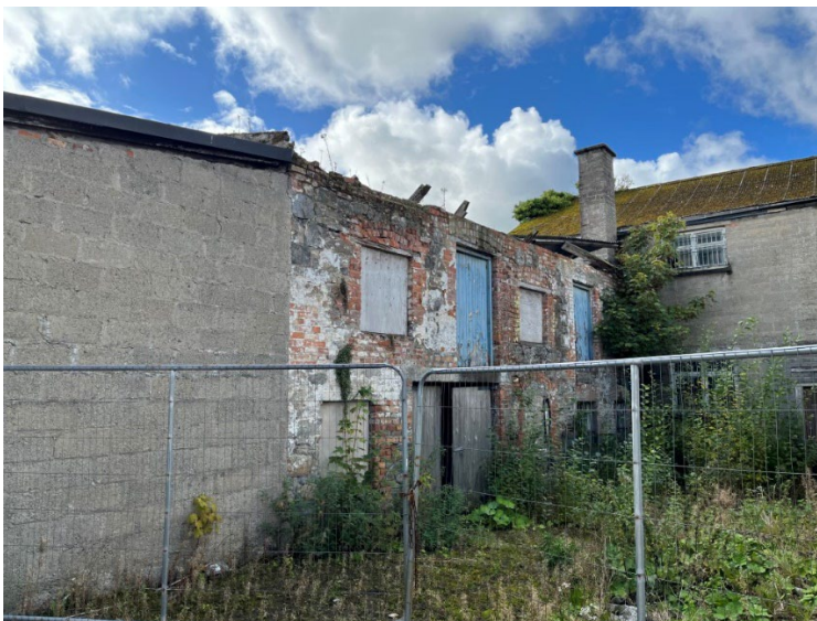
Eastern Wall in Blockwork, A. Collapsed roof over Boiler House, Double door entrance to boiler House Area, C
