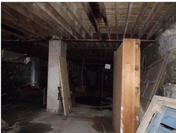
Typical Ground Floor Pier Supporting Steel Beam that Supports First Floor Joists, B
