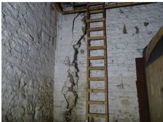
Crack in Northern Wall 2022 A
