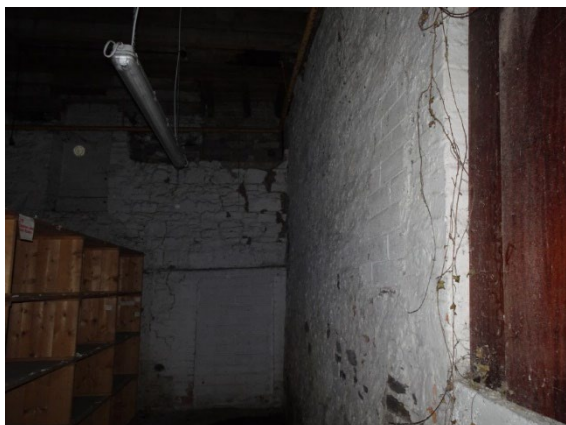
Crack in Southern Wall A
