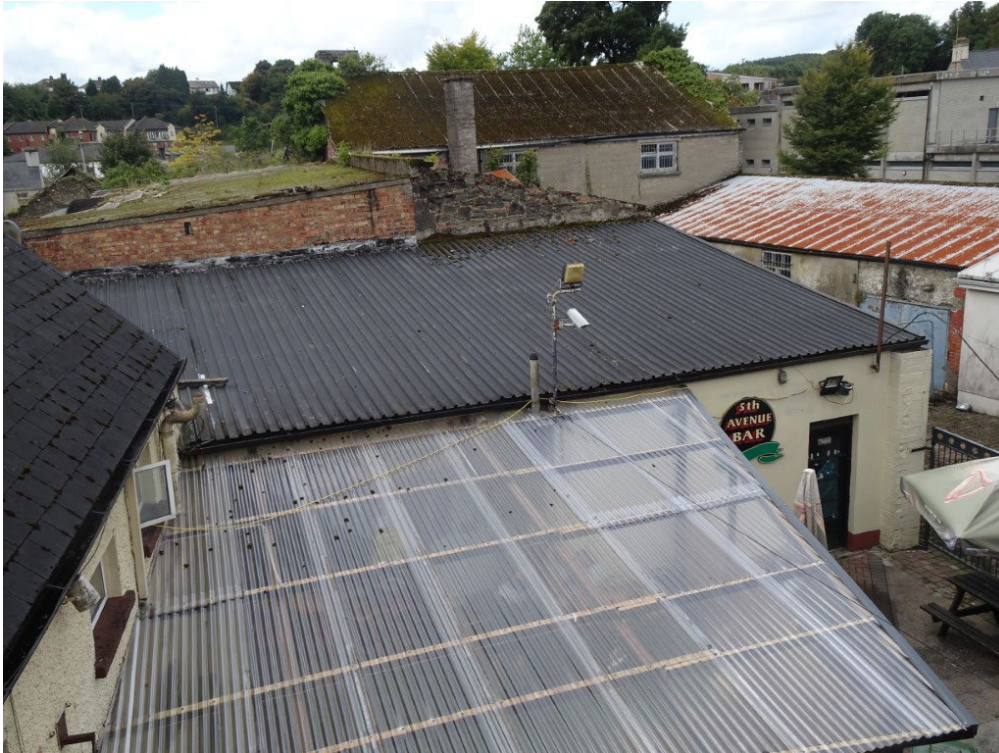
Overall view of Roofs, Duo Pitch Main Building A In the Background, Collapsed Mono-pitch Roof over Boiler House C, note Chimney, Moss covered Flat Roof area B, And mono Pitch Single Storey Area D to the right. Pub in the foreground
