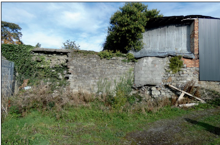
Plate 9: Consolidated building with pcurved wall adjoining southeast boundary wall of Abbeylands public space
