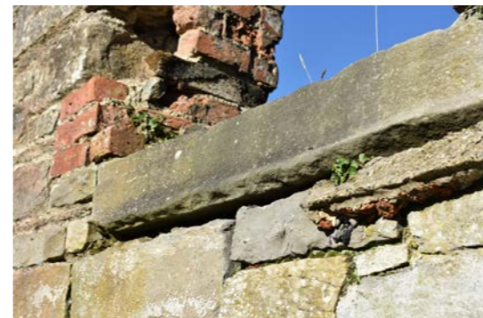
[fig32] 2: Presumed Window Side-Casing re-used as window sill in structure on Donohoe's Foodfare site.
