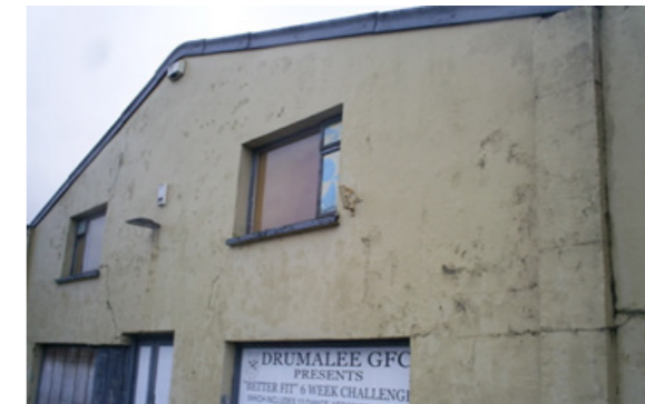
[fig173] Another former commercial building which, being in good order, would be sufficiently warm and dry for bat roosts.
