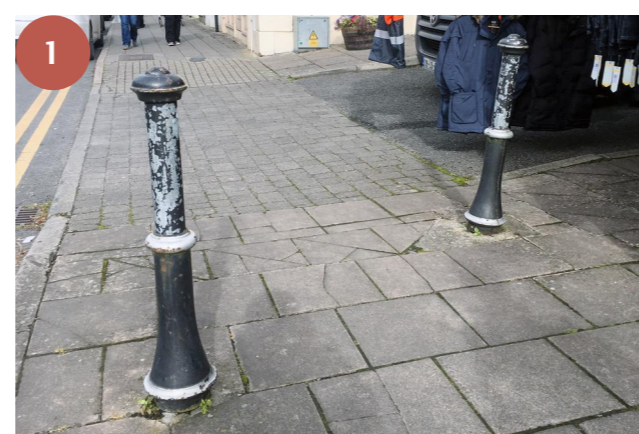
Dilapidated street furniture and paving
